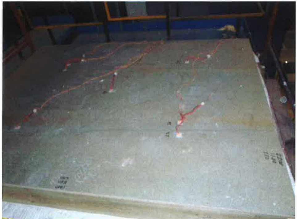
The unexposed face of the ceiling after a test duration of 30 minutes
